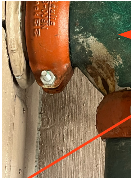
NE stairwell leaking at 4" standard Tee feeding horizontal piping at 3rd floor all sides of tee
